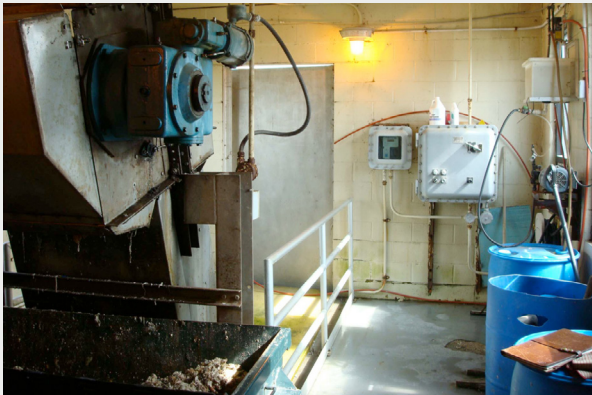
Wastewater Treatment Plant, Headworks with Grit Removal Area
